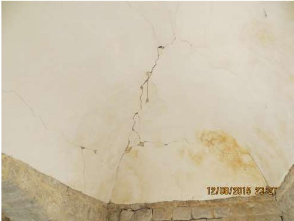
Cracks in the surviving section of the second floor that are a result of the explosion caused by the airstrike.
