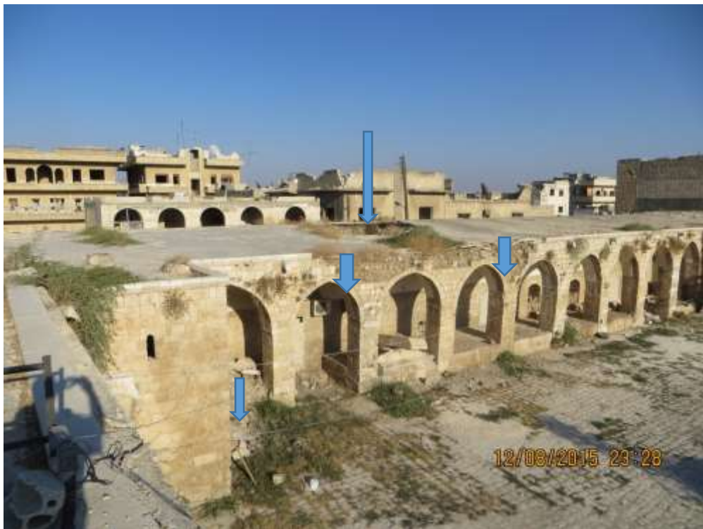
Furthermore, the airstrike caused the large gate at the main entrance to the Khan to come off its hinges and become inoperable. It is currently in need of emergency restoration work in order to return it to use (see images below).
