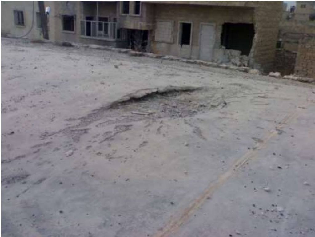
Damage caused by mortar fire
