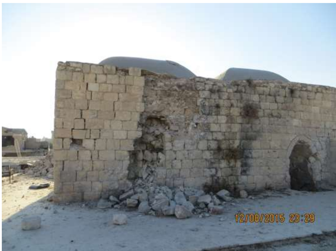
The eastern façade of the second floor showing partial collapse.
