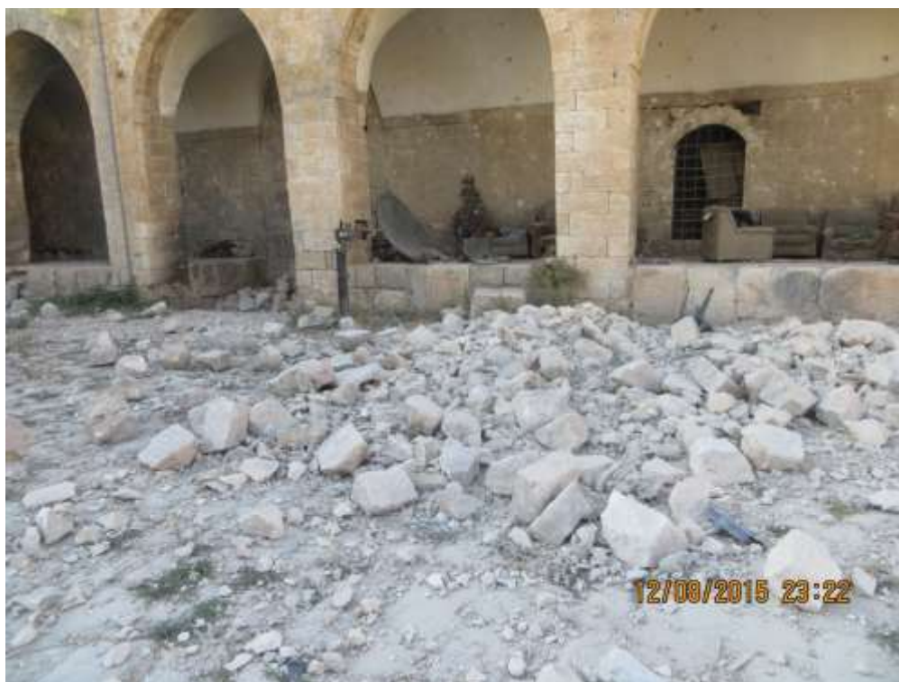
Rubble and stone masonry from the second floor collapsed onto the courtyard.
