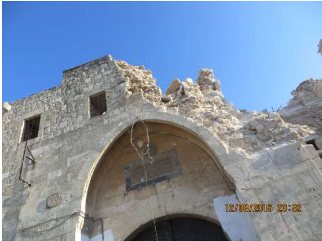
The north side of the second floor showing damage following the latest airstrike
