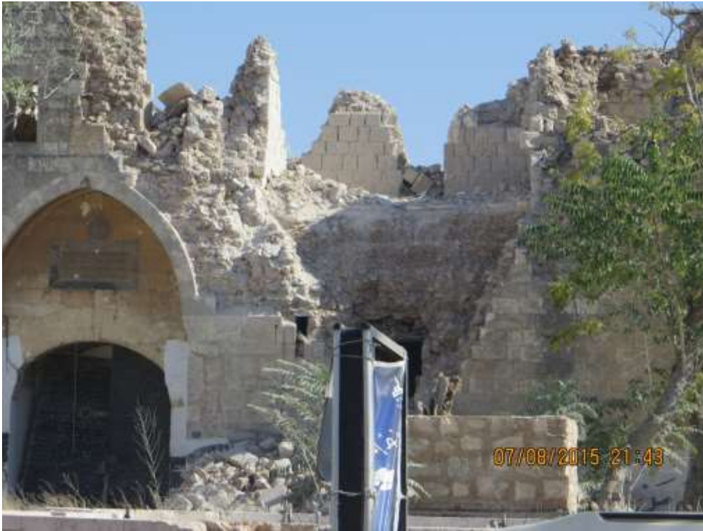
The main entrance from the northern side and the northern façade of the building, which was directly hit with a missile
