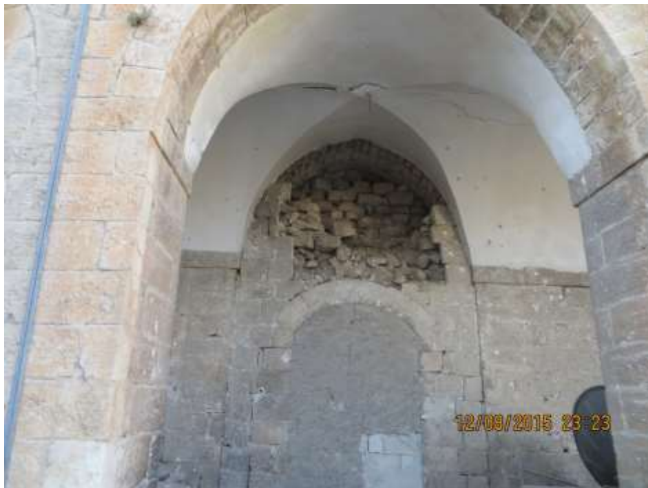
Partial collapse of the first wing as a result of an exploding barrel bomb landing near the Khan
