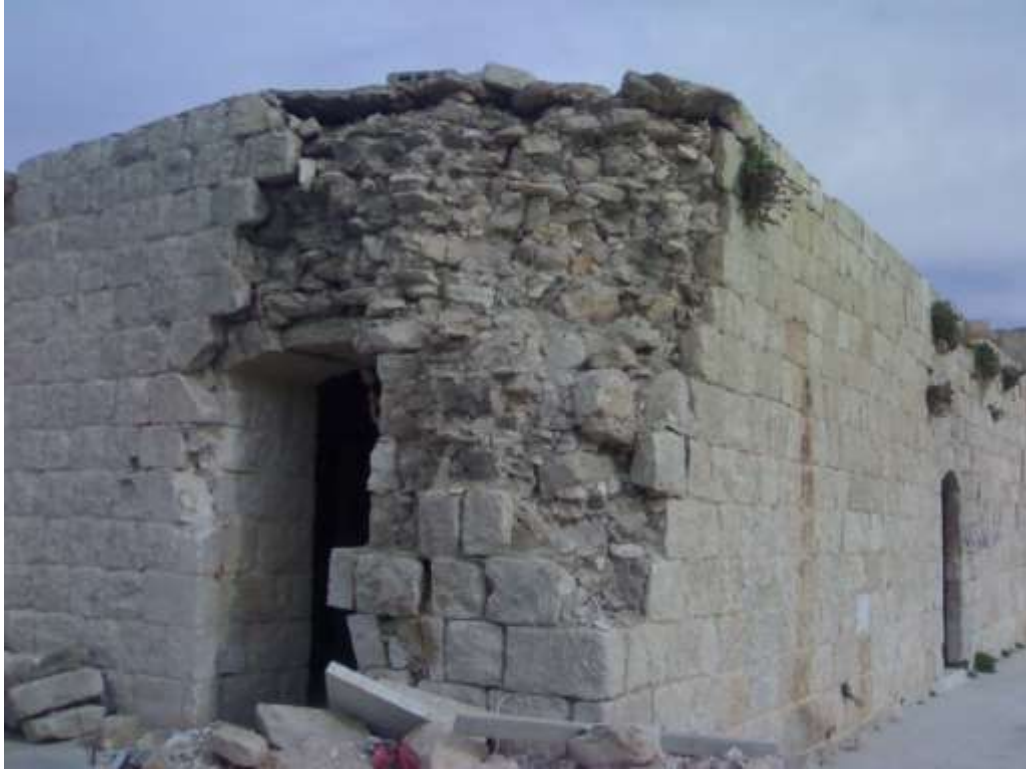
Partial collapse in the southeastern side of the second floor as a result of a missile.
