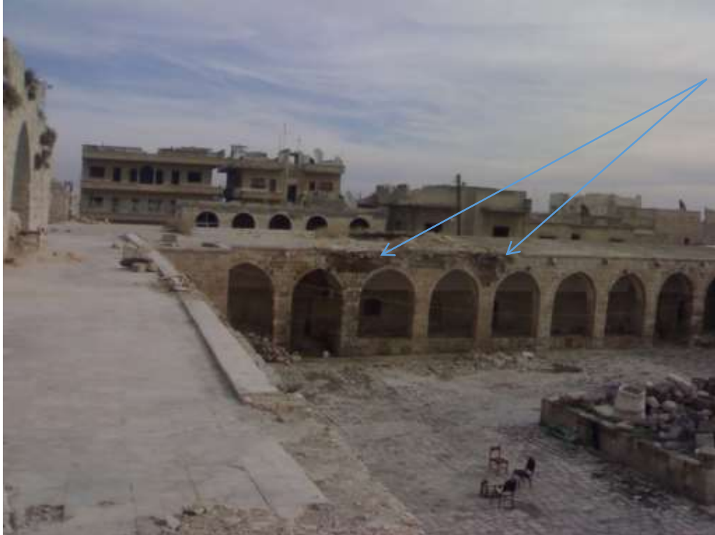
Partial collapse of the corridor on the east side
