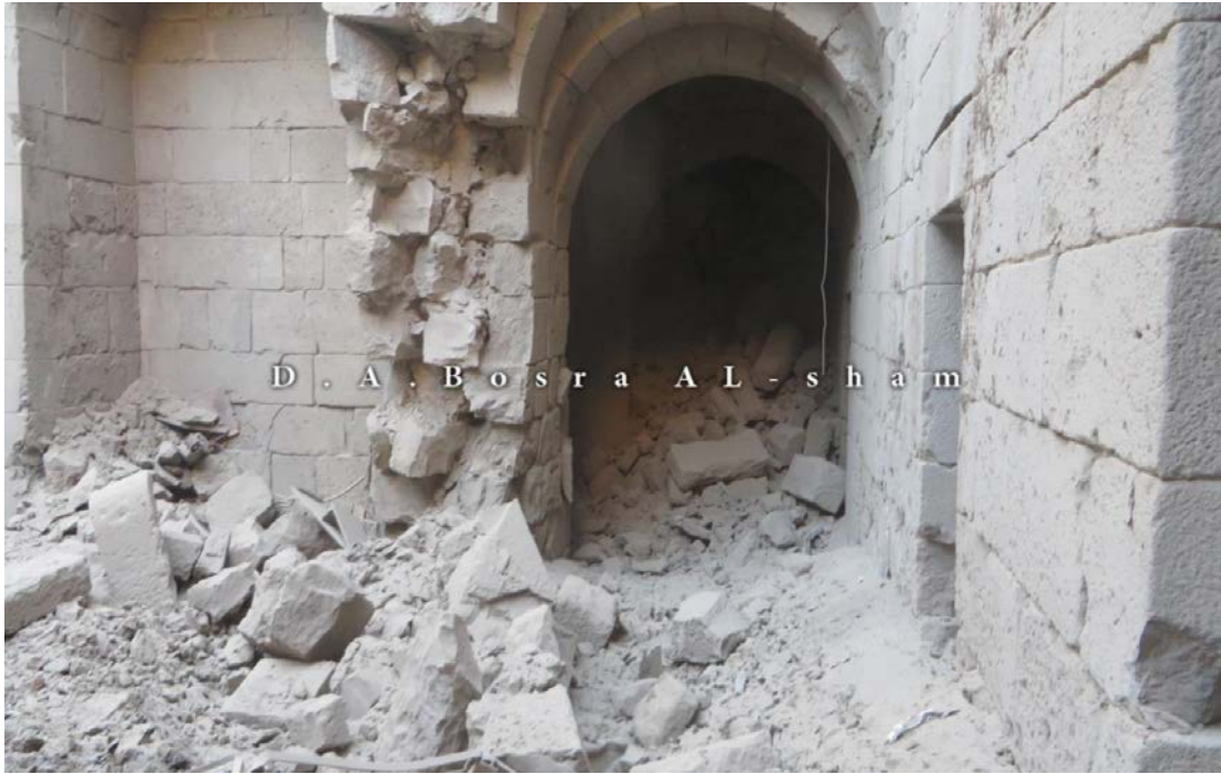
West courtyard after the airstrikes.
