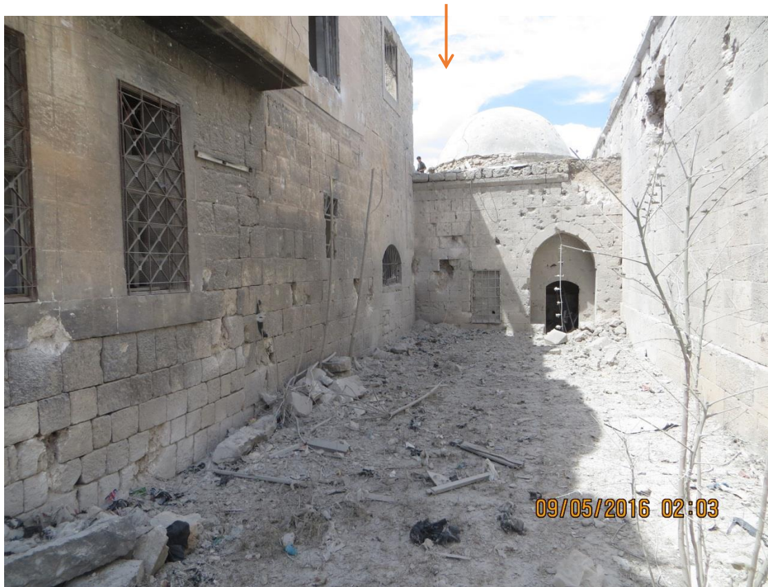
a breach/opening in the external wall of the museum.
