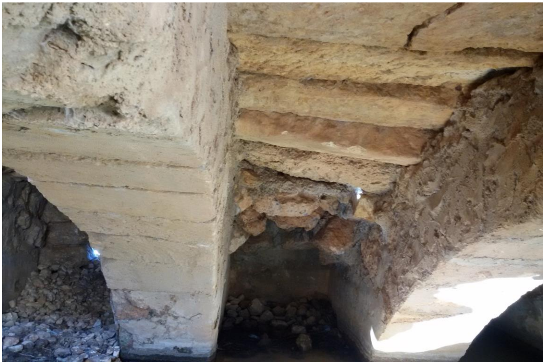
Damage due to weathering and neglect
