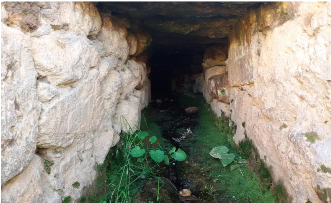
Grass and waste obstructing the main channel
