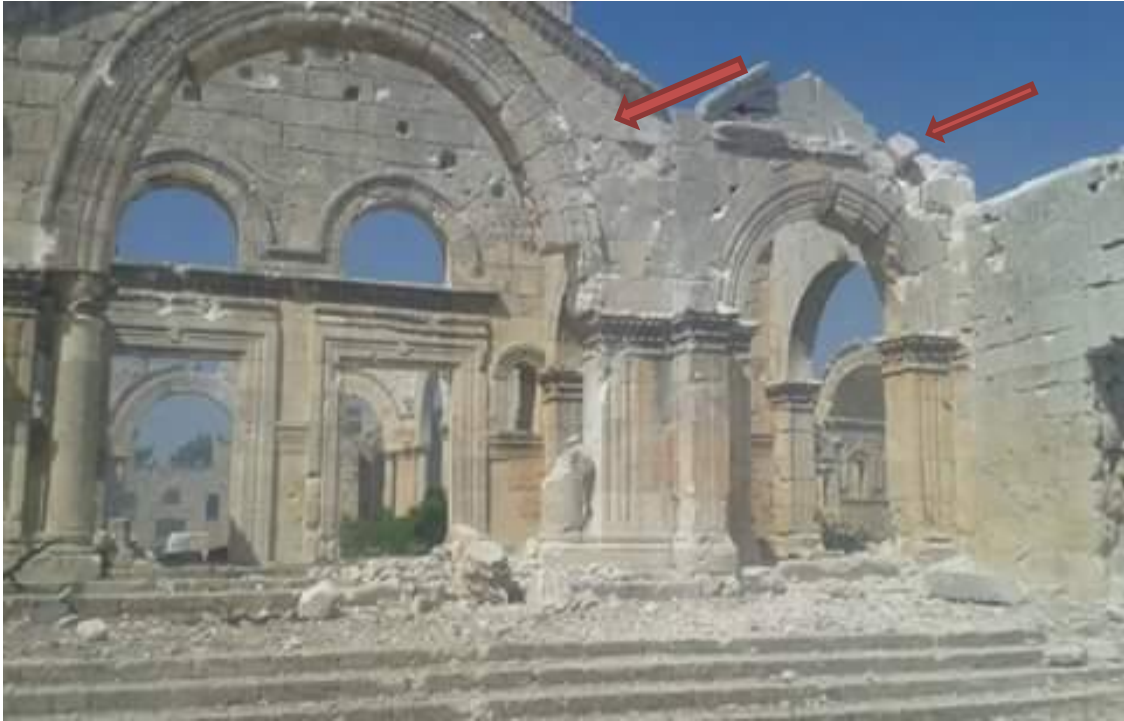
Damaged areas of Simeon Castle after the air strike.
