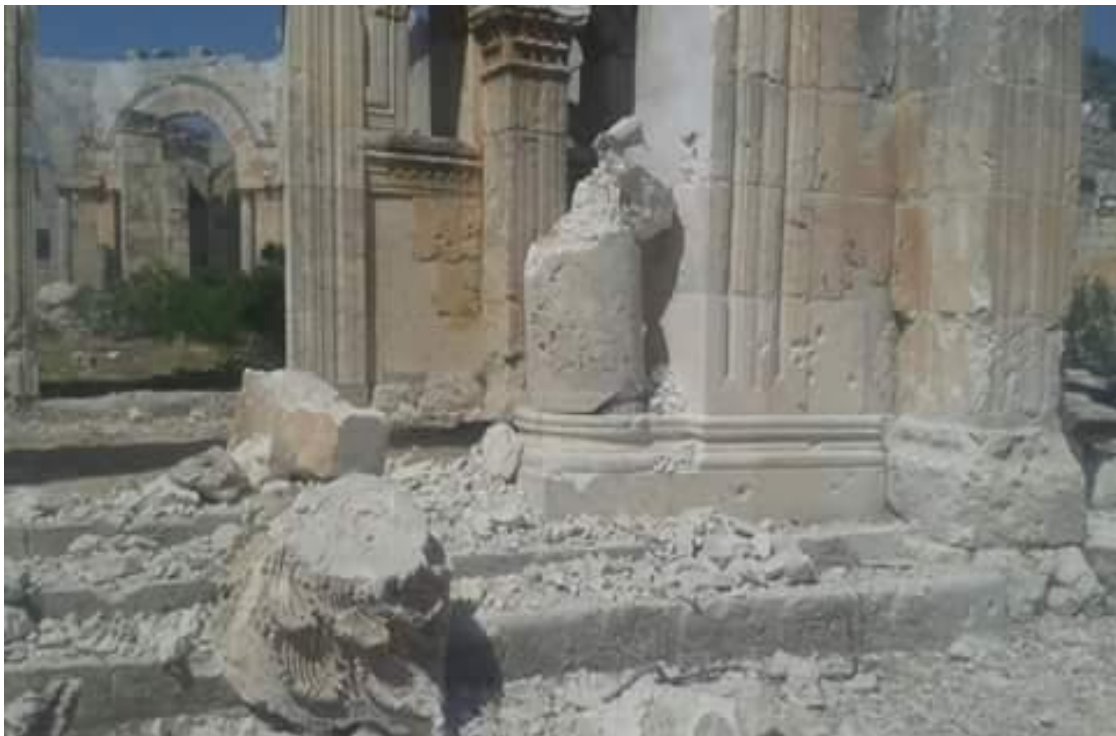
Close up of the damage shown in the photo above.
