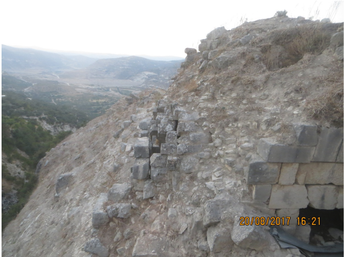
A collapse in the south is a result of weathering and human activity
