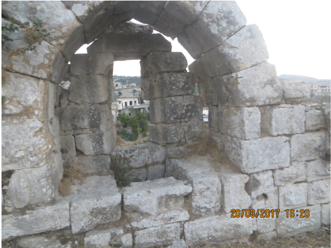
Damage due to weathering effects
