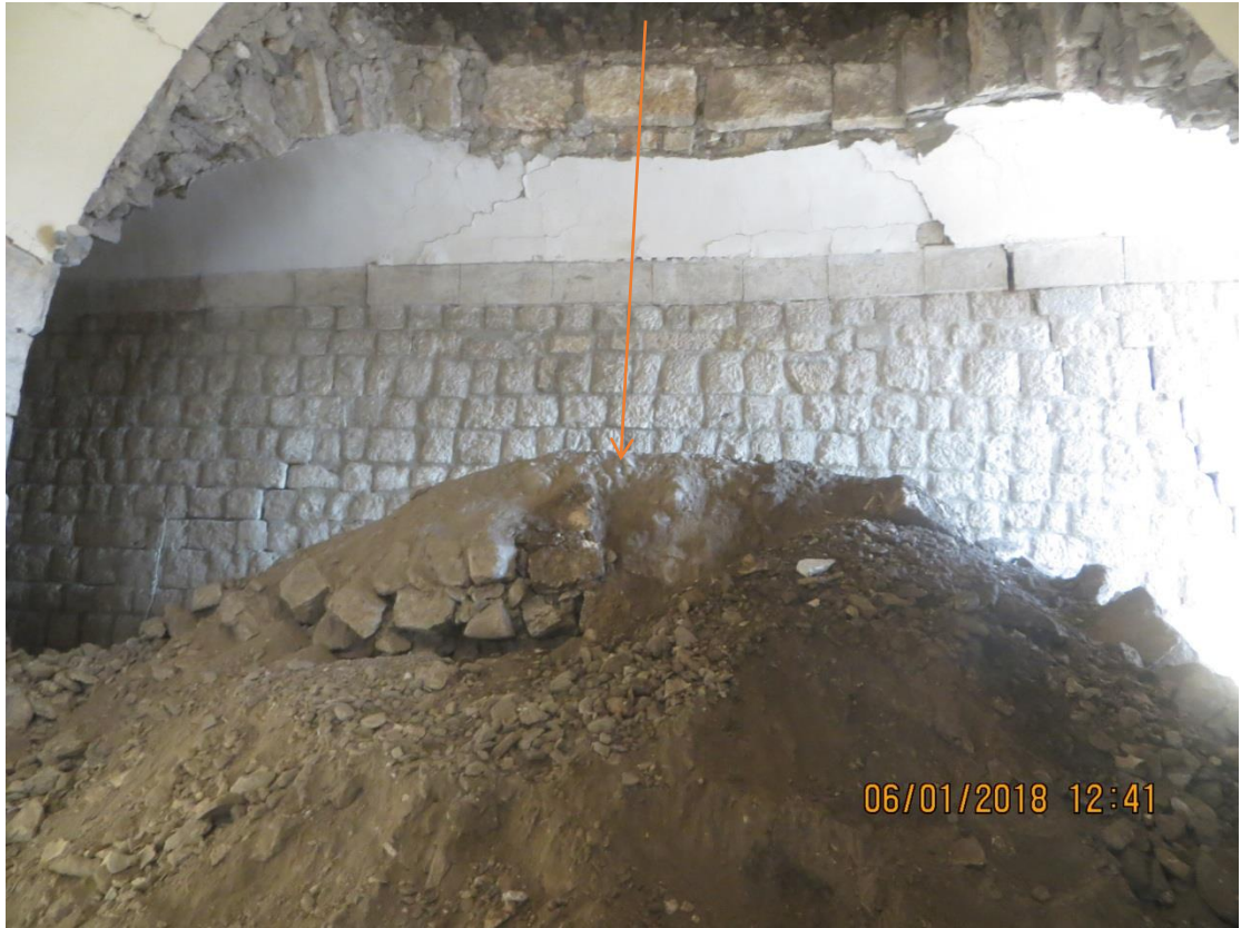
Collapsed roof rubble prior to commencement of work
