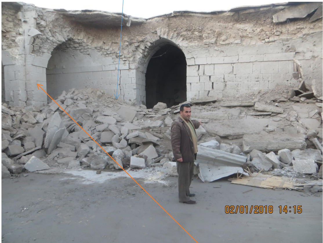
Damage to the northwest corner of the museum
