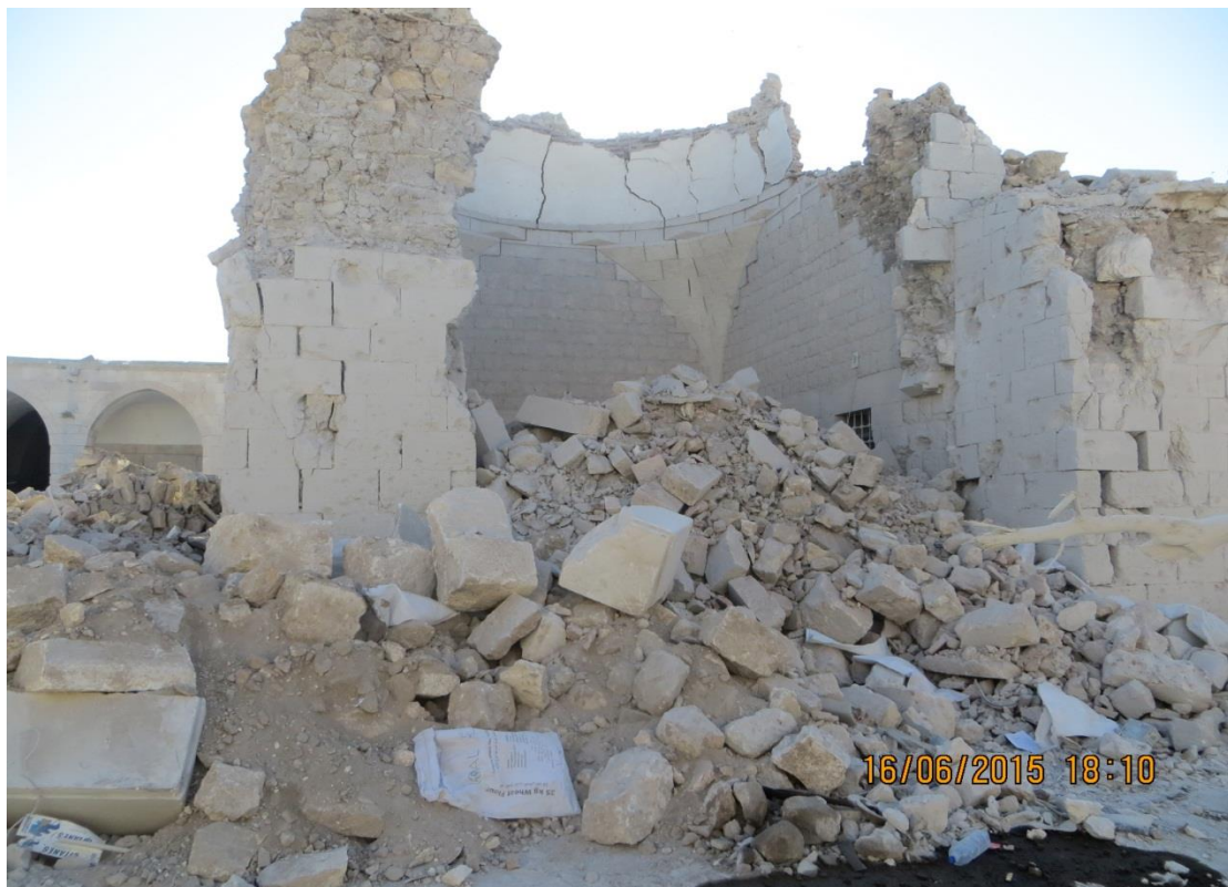
Severe damage to the mosque. The ceiling and the eastern side were completely destroyed and the southern front was partially damaged.
