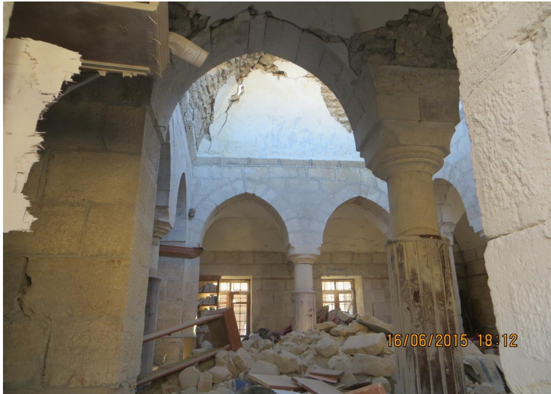
Damage to the Tekkiye . Total collapse of the ceiling and extensive damage of the walls. The Tekkiye contains Al-l'layah Library.
