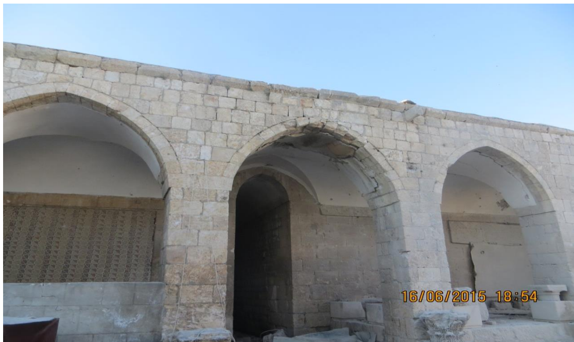
The east wing showing earlier repair done to the arch in the summer of 2014.
