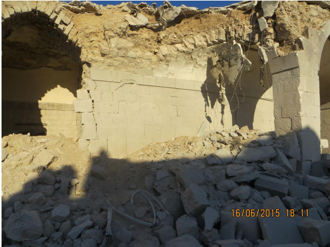
Close up of the severe damage to the covered gallery and parts of the east wing
