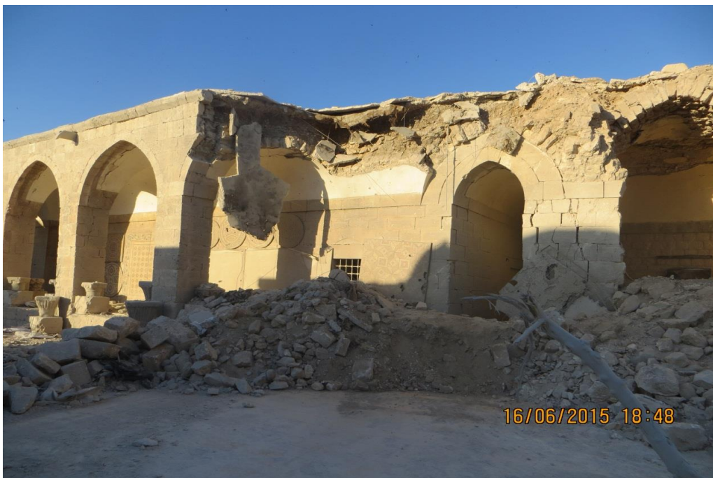
Severe damage to the covered gallery and parts of the east wing
