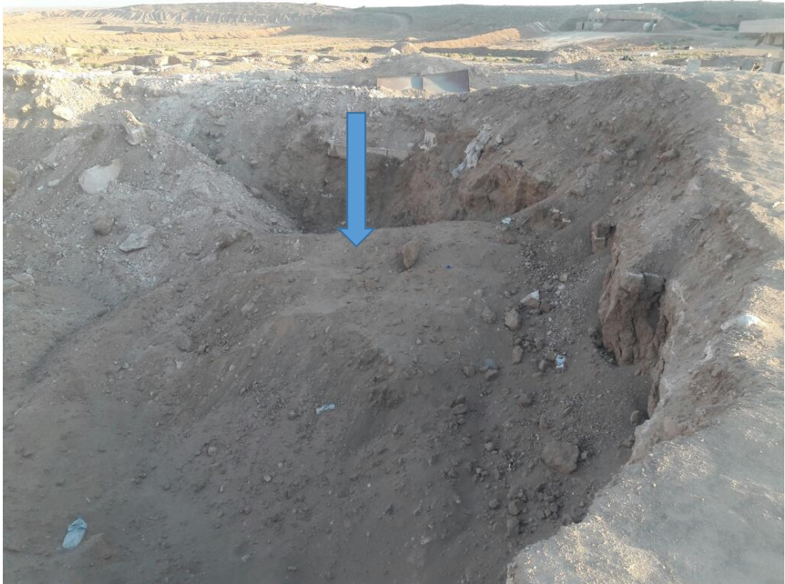
Arrows pointing damage caused by the airstrike and aftermath
