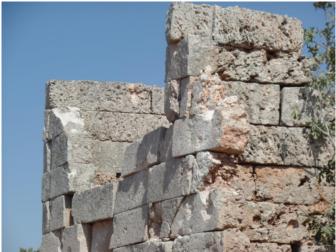
Severe damage to the wall
