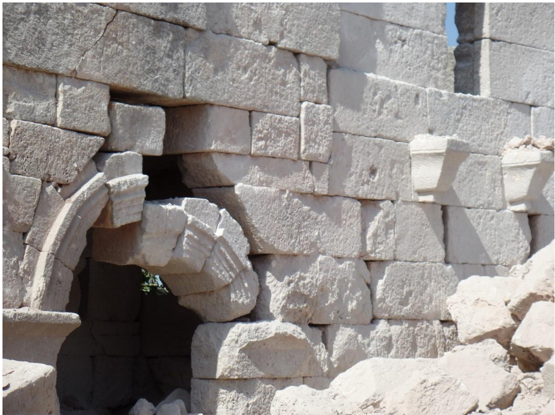
Severe damage to the walls and the need for emergency intervention and repair work
