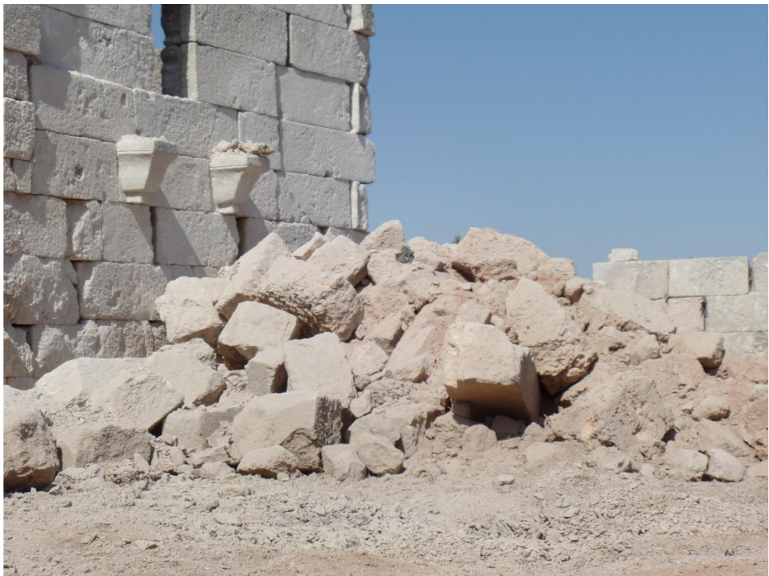
Collapse of the entire archaeological building
