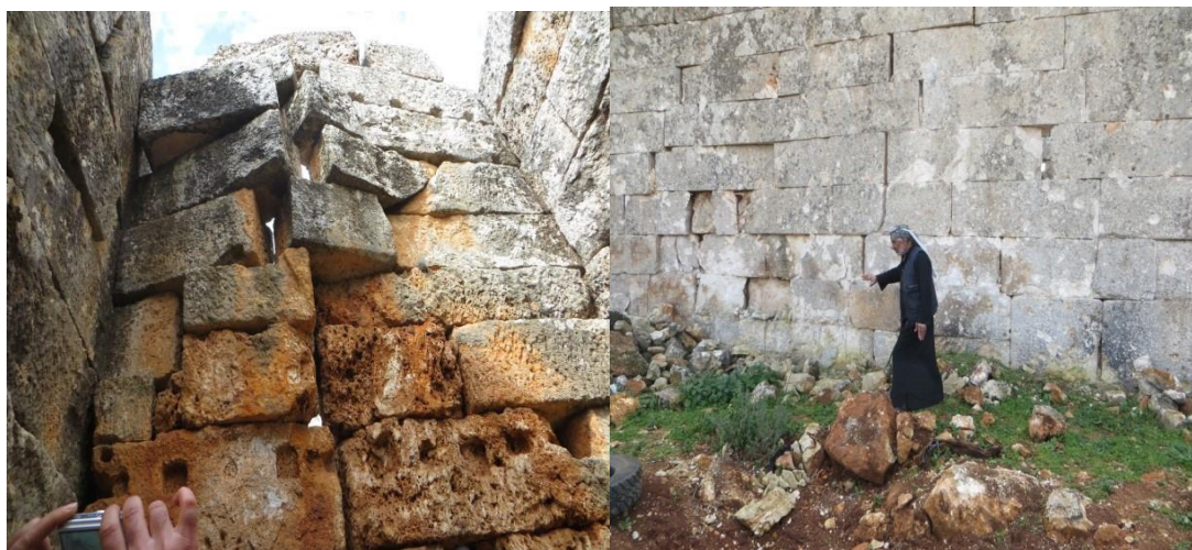
Damage caused by previous attacks by Syrian regime bombing in 2013
