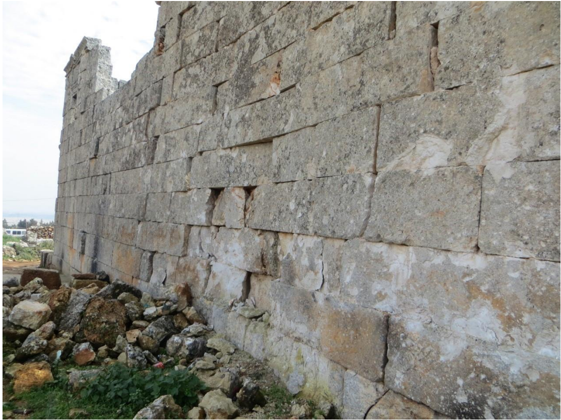
Damage caused by previous attacks from Syrian regime bombing in 2013
