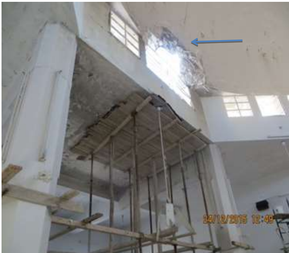
Airstrike targeted the base of the mosque's dome from the east side.
