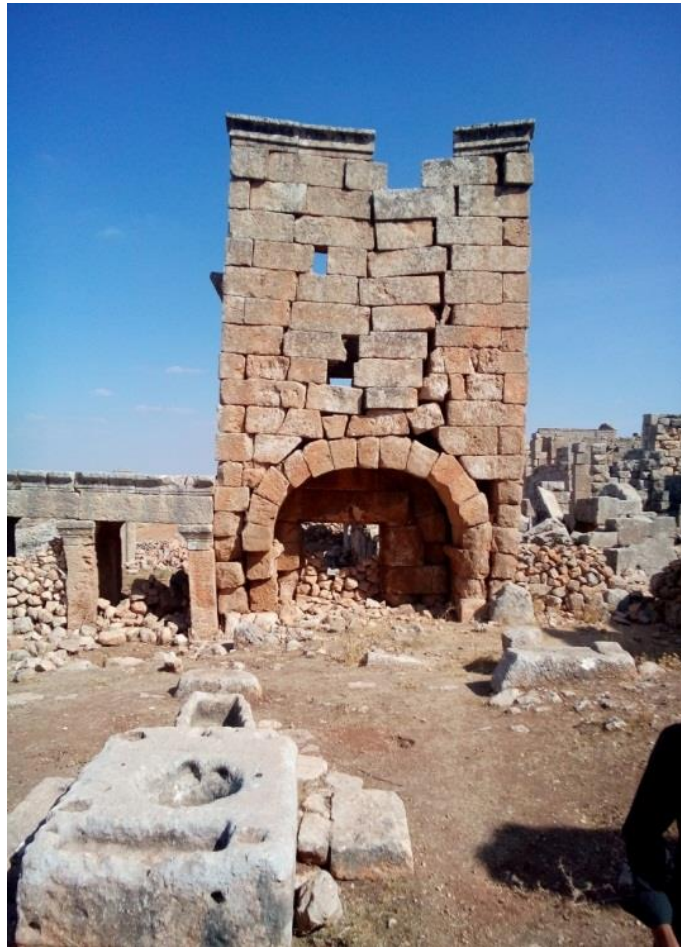
Damage caused by neglect
