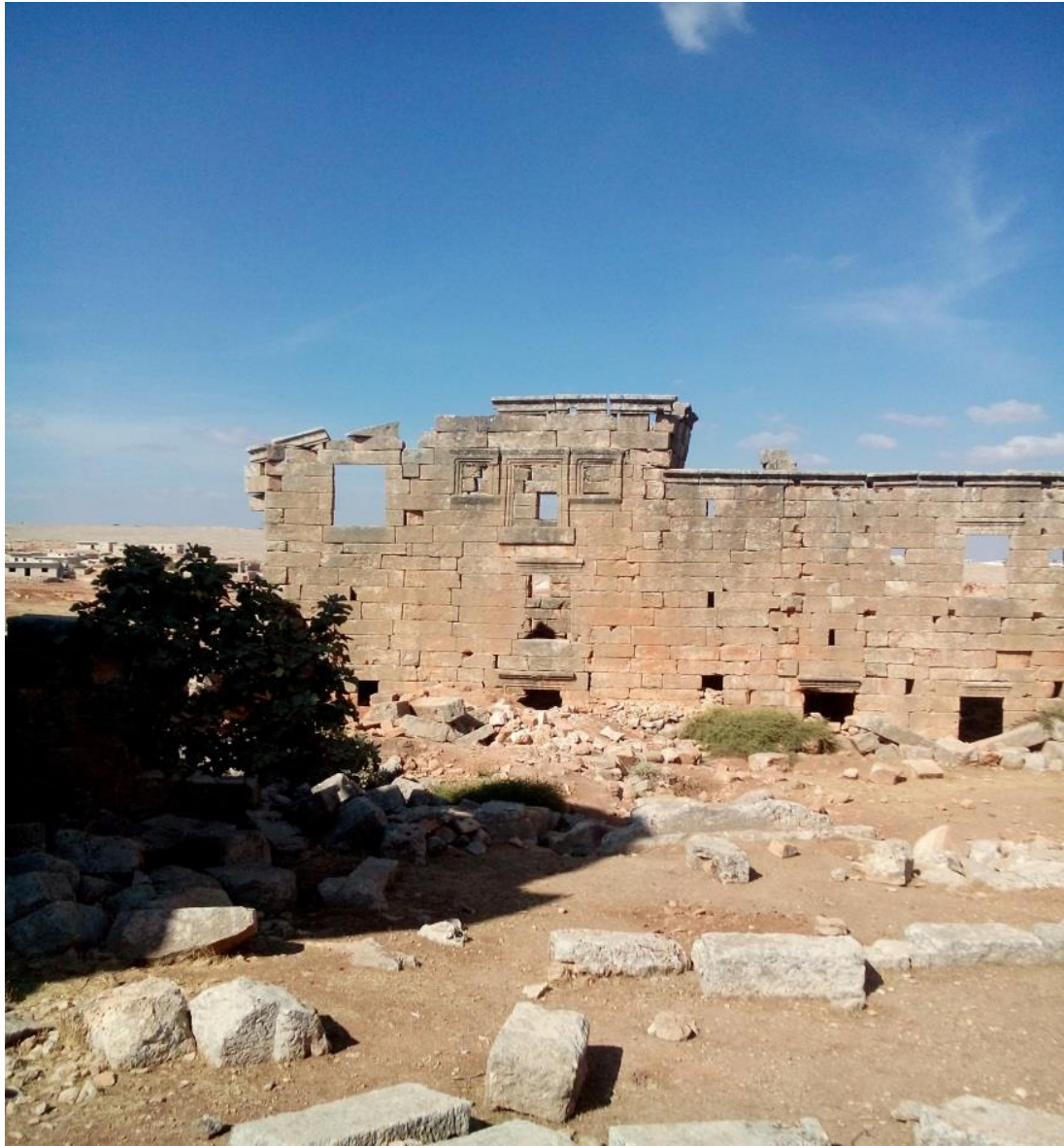
Illicit digging at the site and near to the walls causing damage to buildings and foundations
