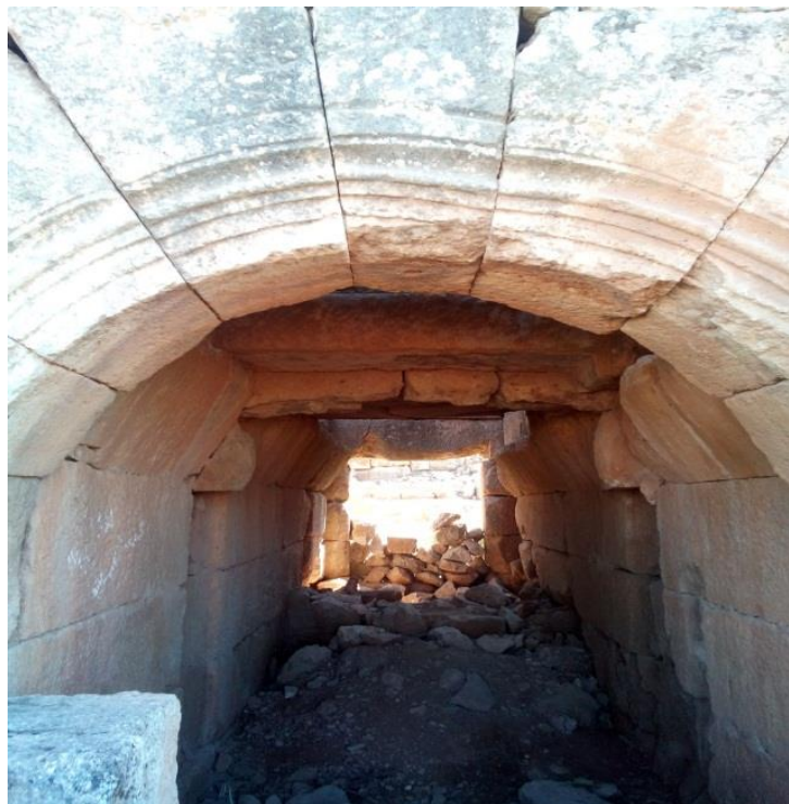
Damage caused by neglect
