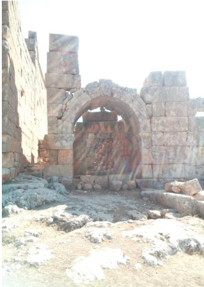
Damage caused by neglect
