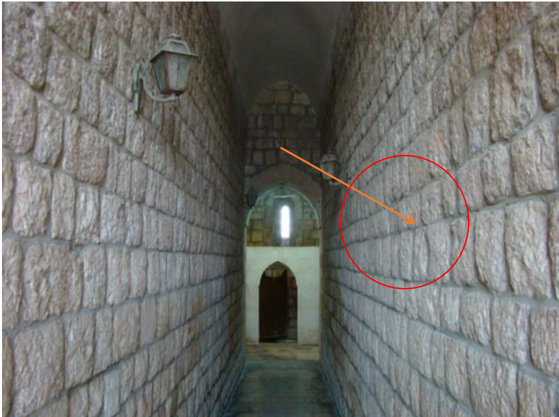
Wall prior to damage causing deviation
