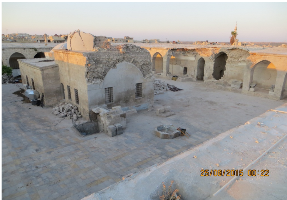
South side of the mosque (facing north east) prior to removal of the dome.
