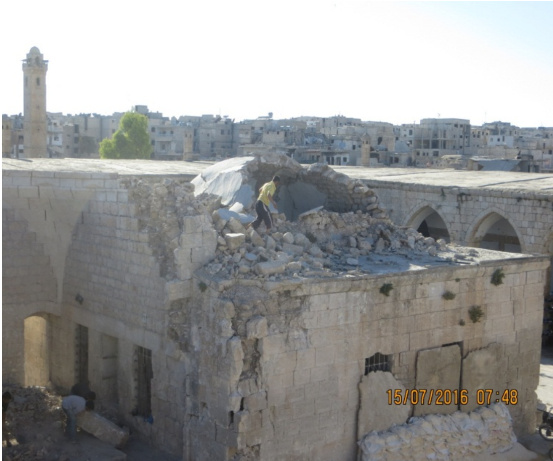
View of the damaged dome of the Tekkiye
