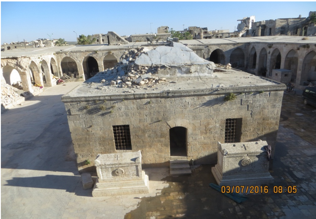
North side of the mosque (facing south) prior to removal of the dome
