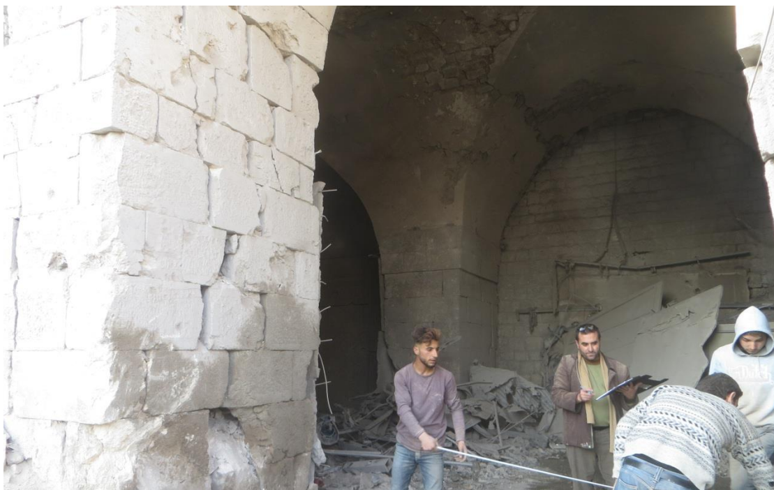
Documenting the damage
