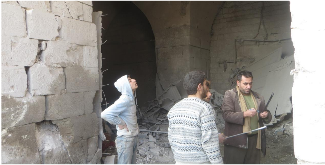
Documenting the damage
