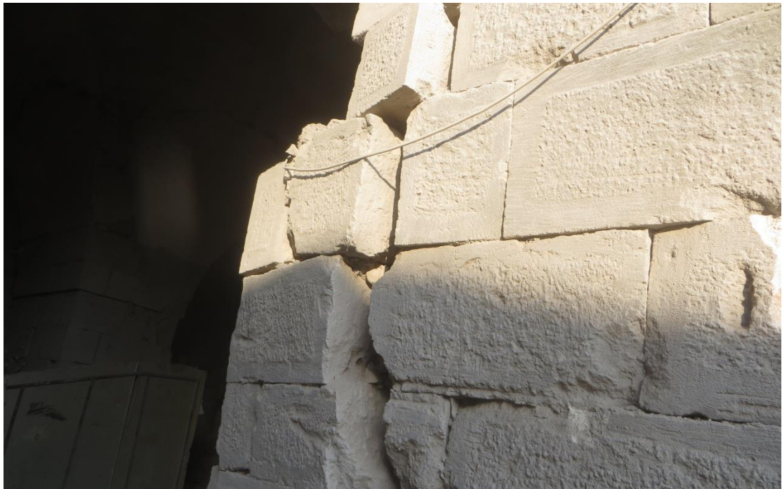
Documenting the damage
