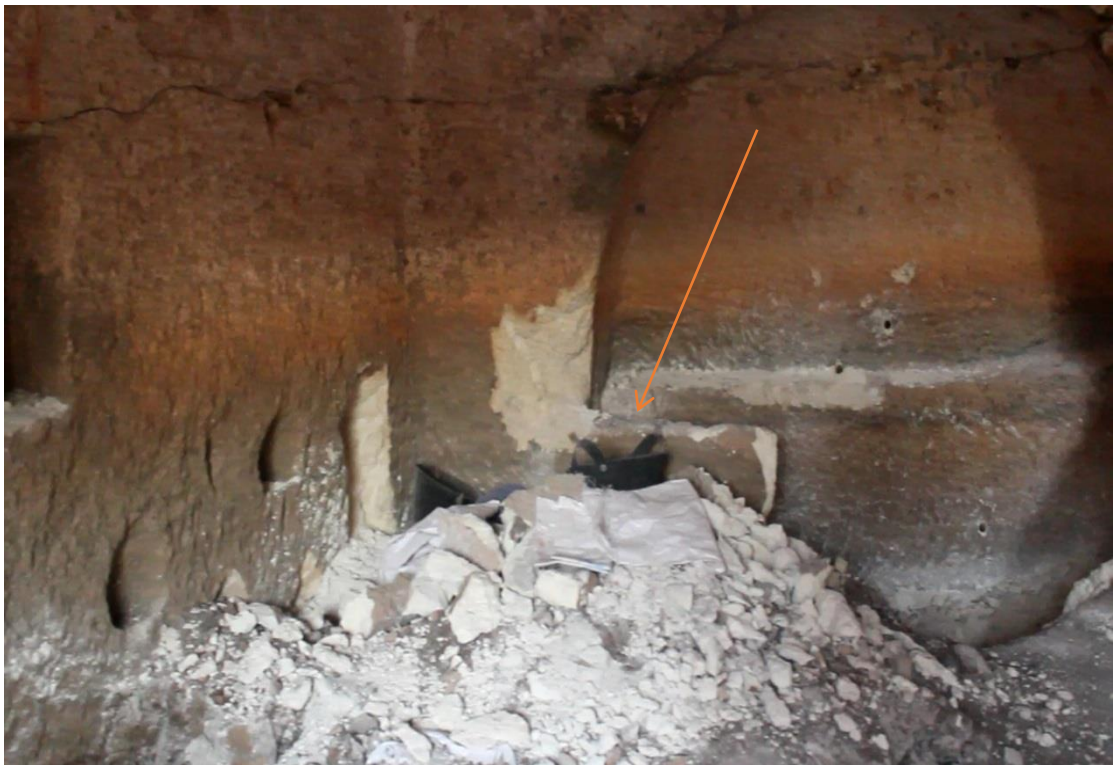
Illegal excavations inside the building
