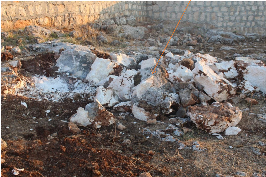
Damage caused by breaking up masonry
